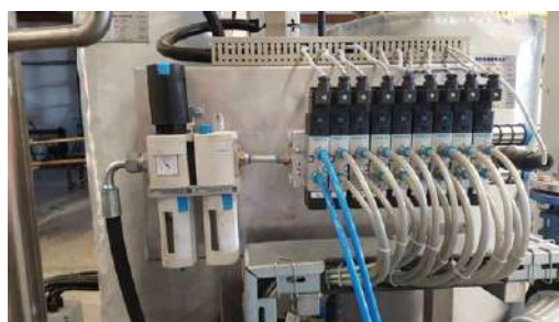
Pneumatic Control System
