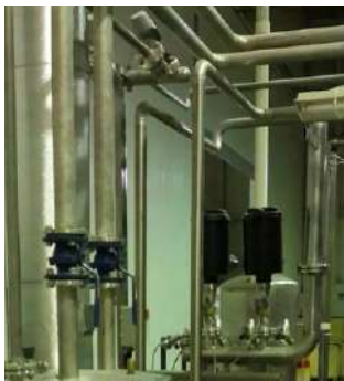
Pipe and EO Gas Connection System
