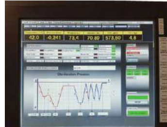
HMI Display, SCADA Software
