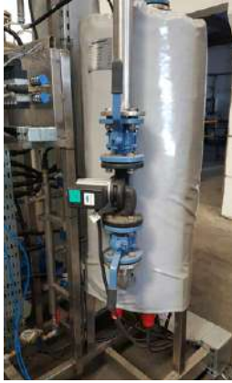
Water Heating Tank and Hot Water Recirculation System
