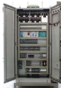
Electrical Panel, PLC, Sensor System (Temperature, Humidity, Pressure, etc. Safety Sensors), Electronic Equipment
