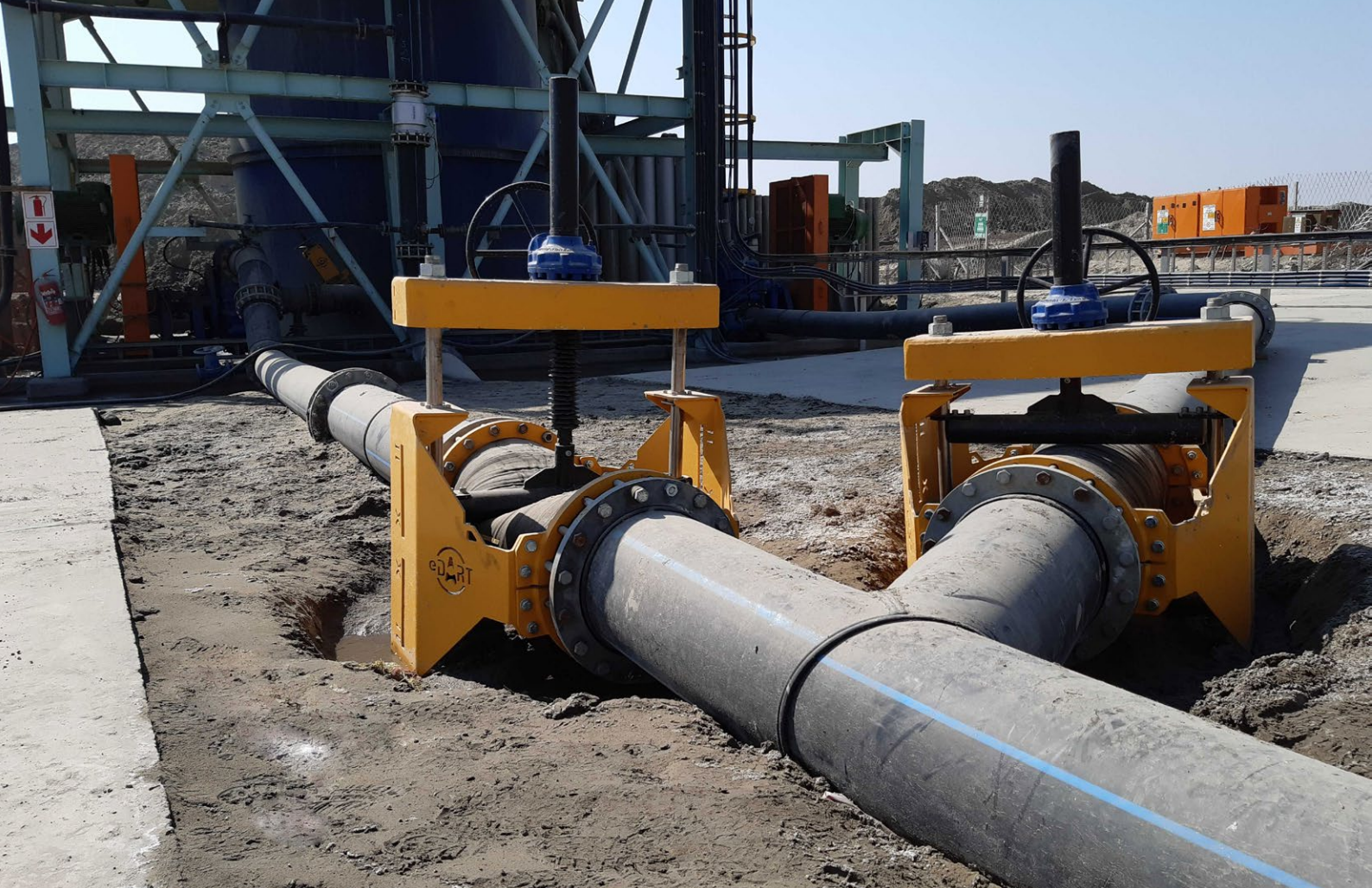
Manual open frame pinch valves used on the line to the tailings facility
