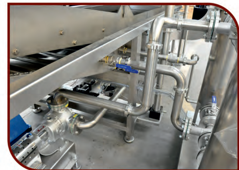
OIL CIRCULATION SYSTEM (OIL AUTO FILTRATION PUMP)
