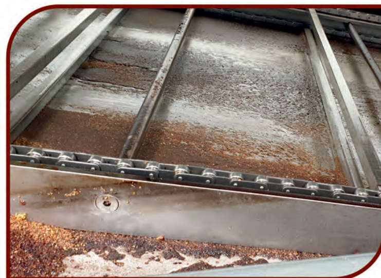
SCRAPER (INSIDE BOILER DUST AND PARTICLE CLEANING SYSTEM)
