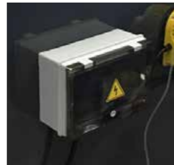
Unloading system stopper box.
