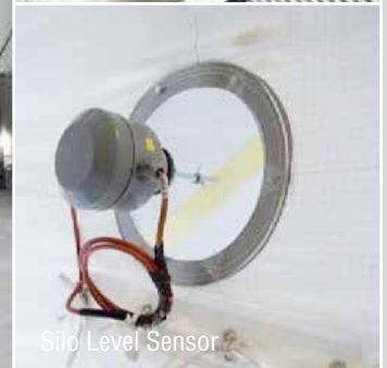
Silo Pipe Switch
