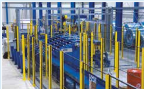
Impianto completo Complete plant
